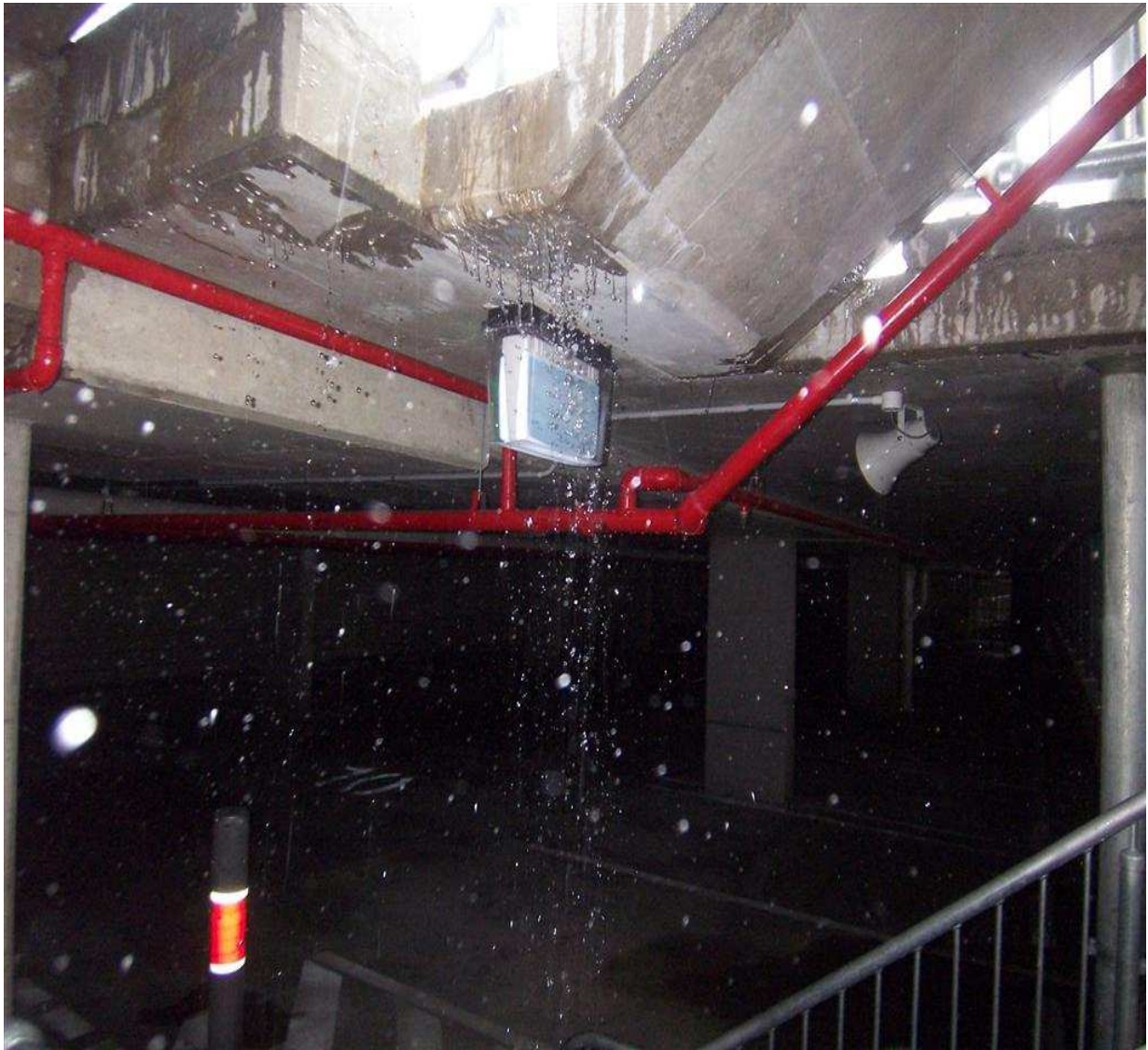
Rainwater entering car park
