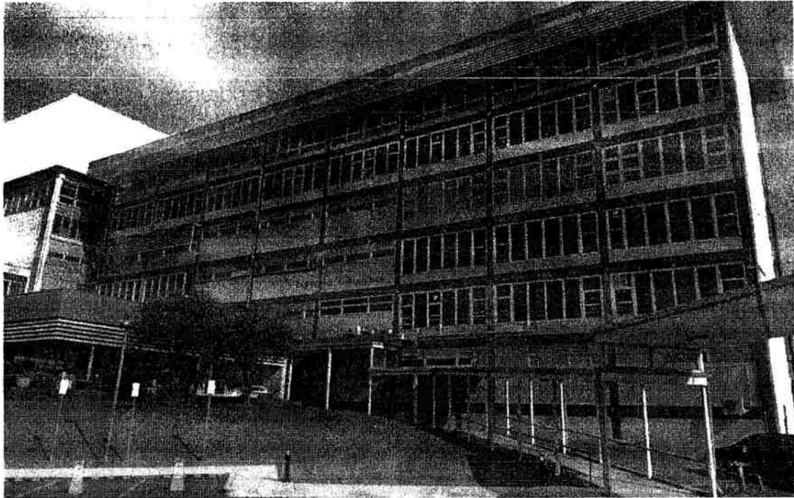
Eastern facade view: Pink area found loose brick work and yellow area small section of loose aluminium which was removed.
