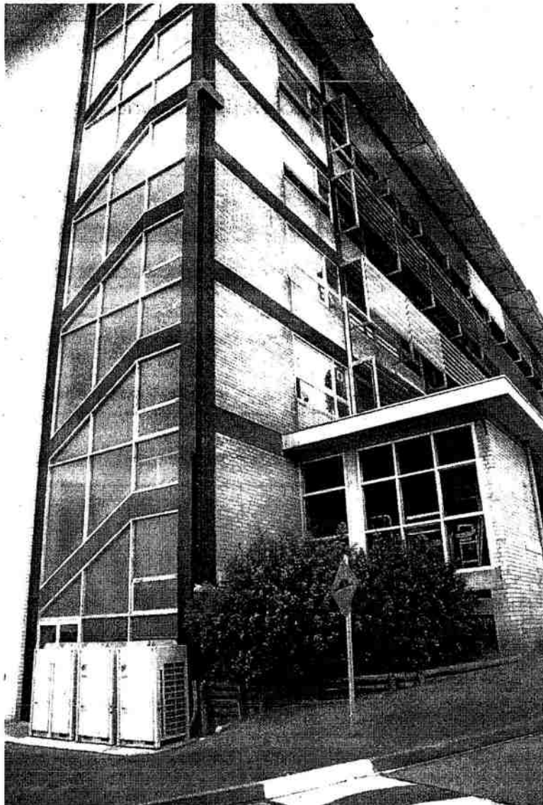
Image 15 - Continuation of Northern Elevation where it meets the Western Elevation showing grass area below.
