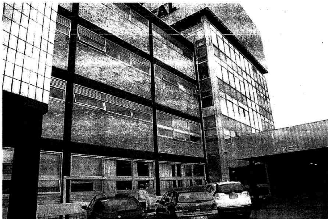
Image 8 - Closer view of Southern Elevation directly above cars parked below near the entrance of the tower section of the building.
