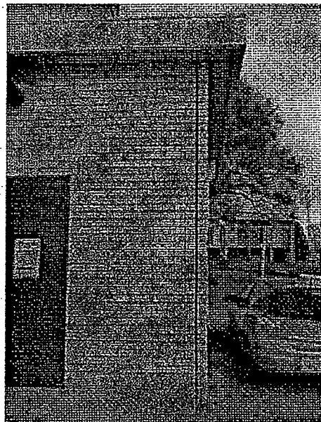
Figure B1-15: Brickwork – Gradual leaning and peeling of brickwork panel. Ground level, northwest corner of west wing.
