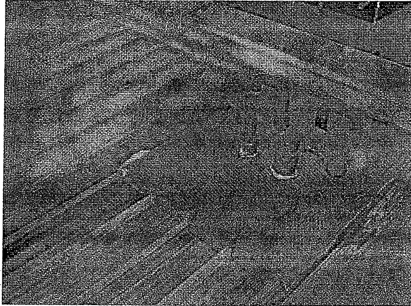
Figure B5-5: East wing: Severe corrosion present on roof sheeting of the western wing likely due to bimetallic action.
