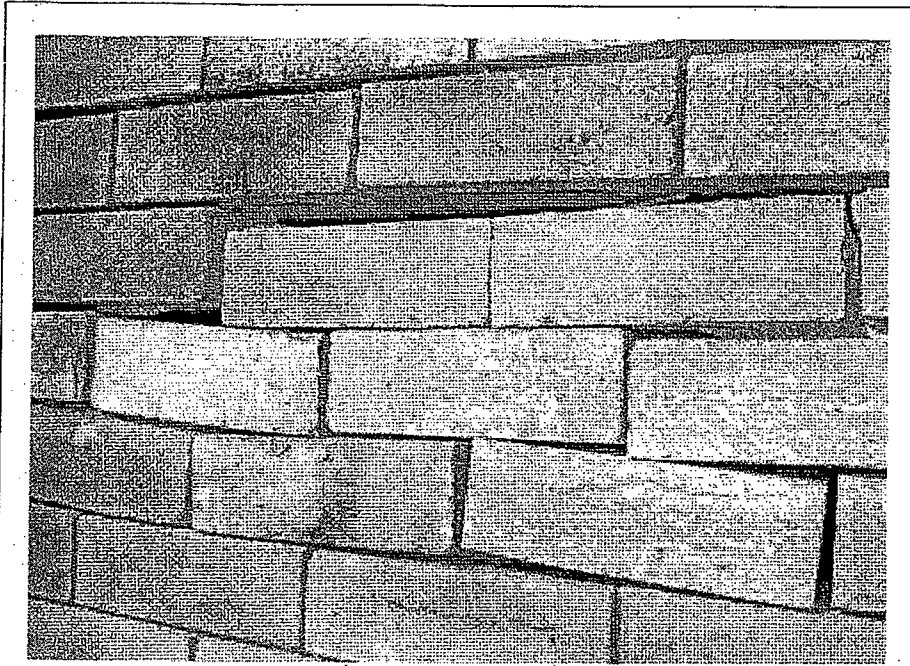
Figure B1-25: Brickworks – Erosion of mortar resulting in brickwork displacement and loss of structural integrity.
