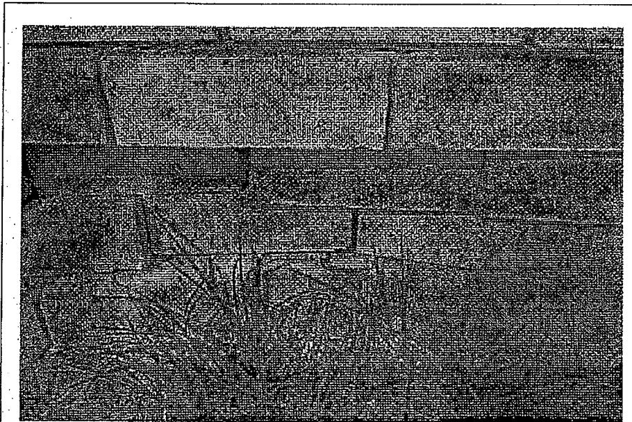
Figure B1-20: Brickwork – Displacement of brickworks due to loss of mortar and impact loads on the northern wing.
