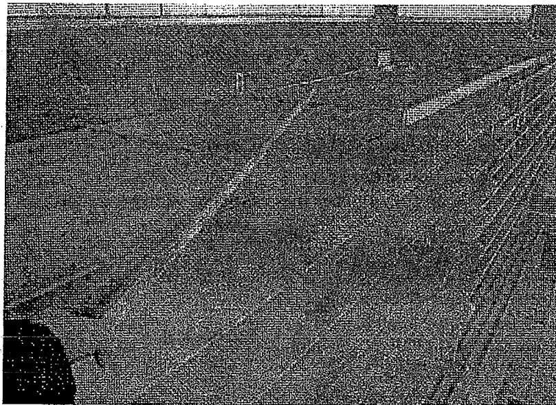
Figure B3-2: Sunshades – Loose and corroded sunshade louvre systems.
