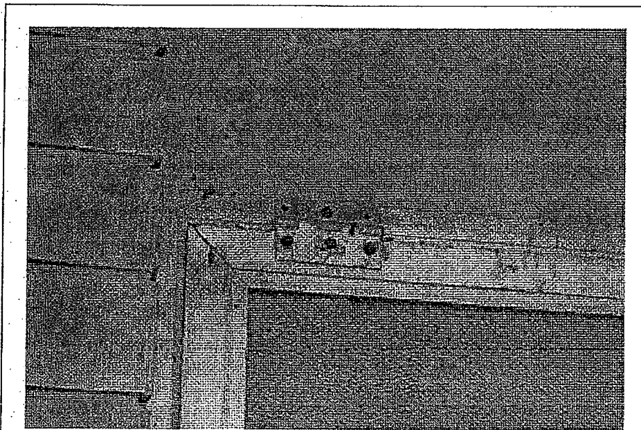
Figure B2-10: Windows and Louvres – Corrosion and missing window hinge screws.
