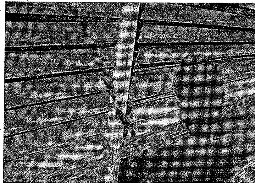
Figure B2-2: Windows and Louvres – Pitted edges and dislodged louvre fixings.
