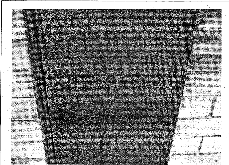
Figure B4-7: Rendered Beams & Columns – Damaged render columns.
