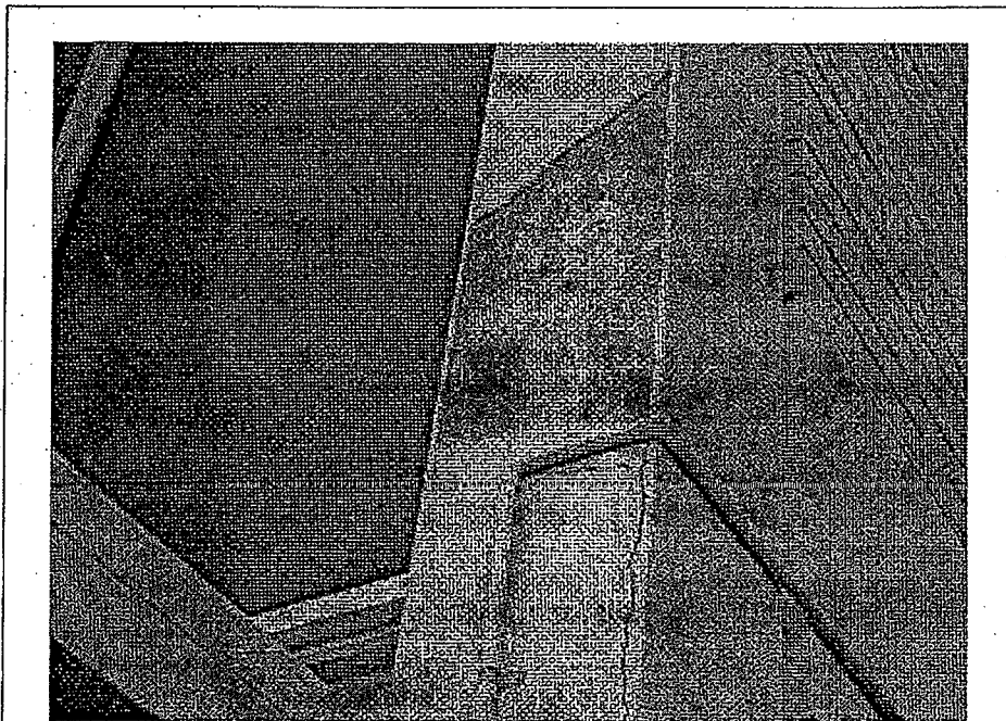
Figure B4-8: Rendered beams & columns – Damaged rendered
