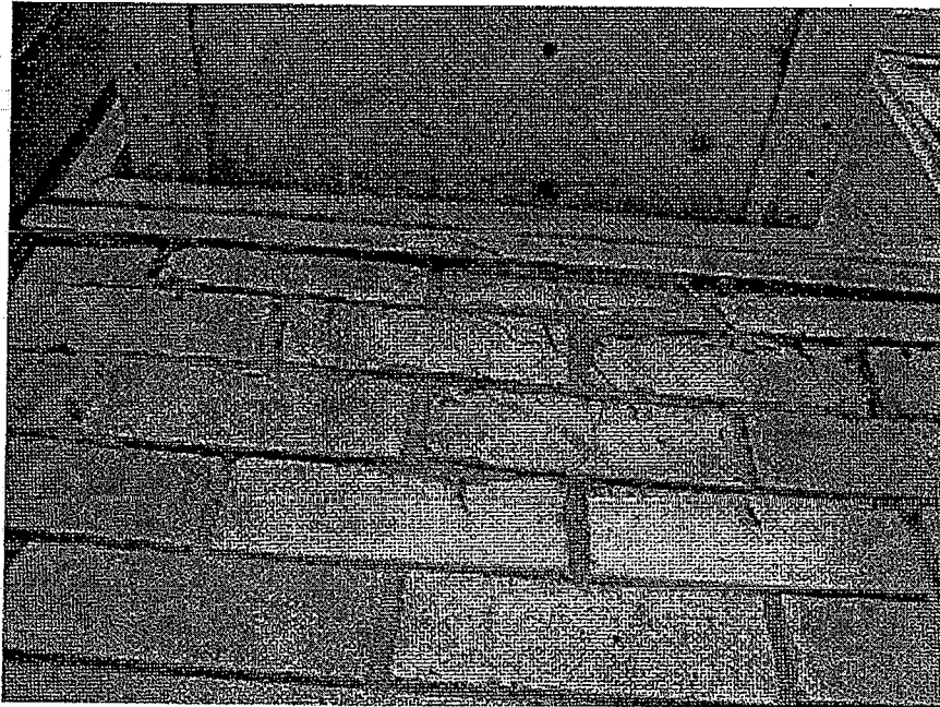
Figure B1-22: Brickwork – Inadequate silicone application to brickwork mortar joints.
