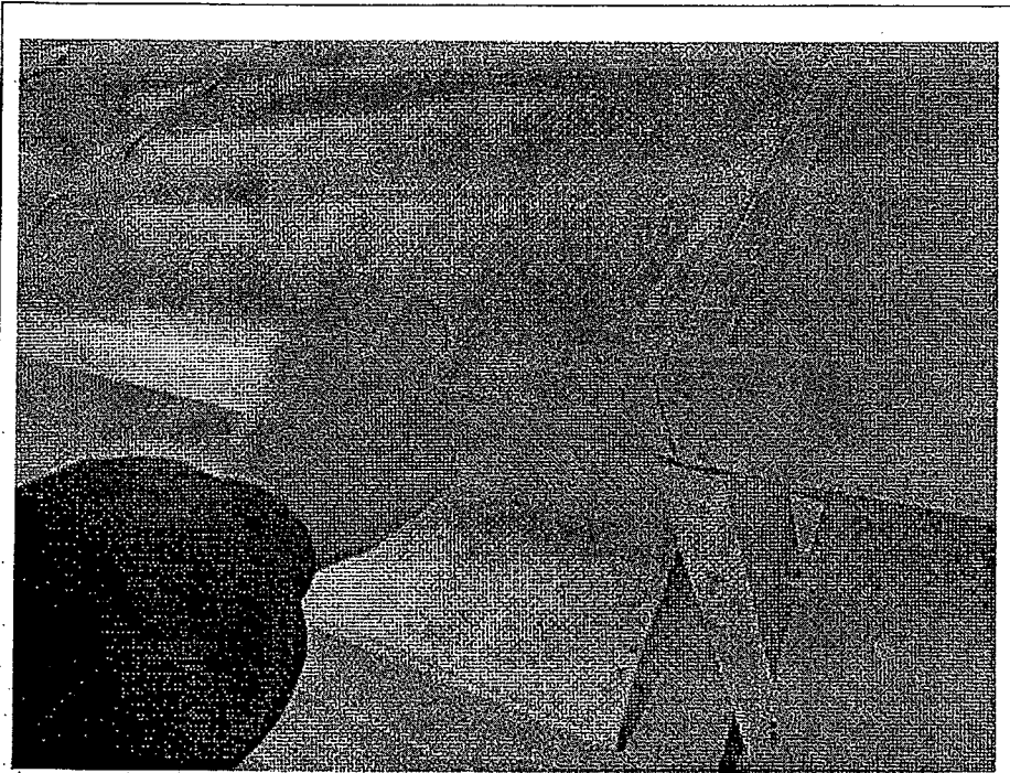
Figure B3-3: Sunshades – Loose and corroded sunshade fixings.
