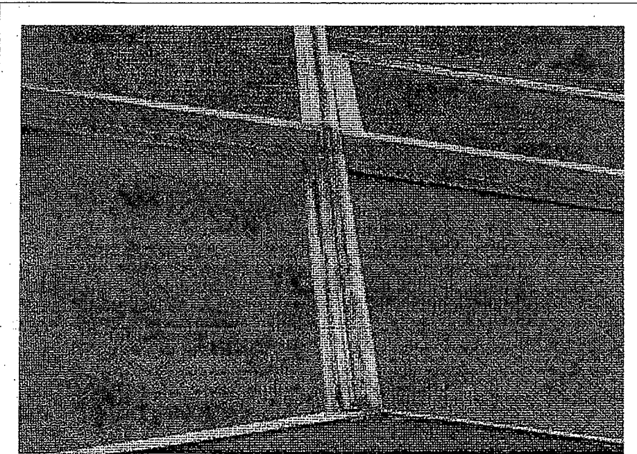
Figure B2-20: Windows and Louvres – Displaced trims on curtain wall stairs windows.
