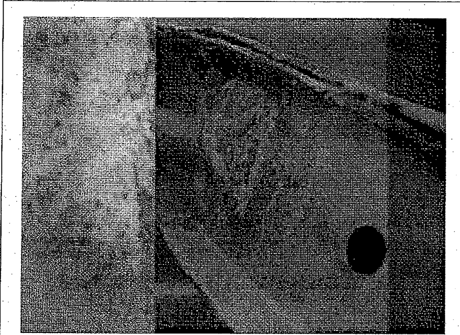
Figure B3-9: Sunshades – Pitted sunshade edges and corroded sunshade fixings.
