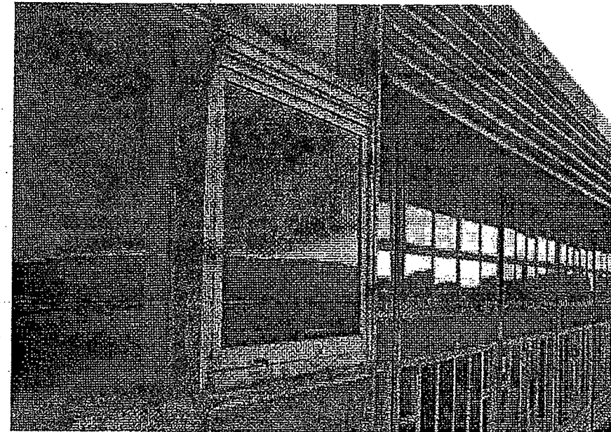
Figure B2-12: Windows and Louvres – Glazing film deterioration on new window panels on western wing.
