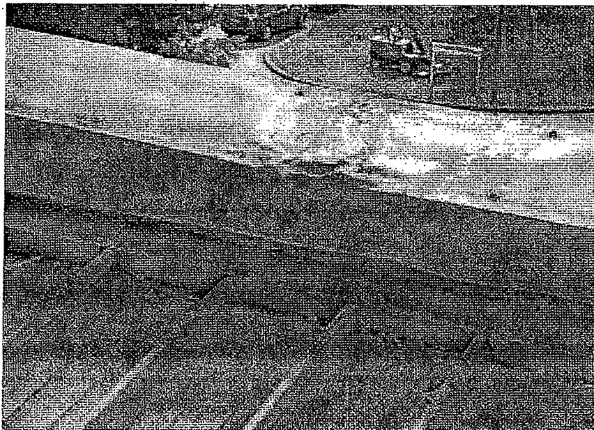
Figure B5-7: Roof areas – Damaged parapet capping on the western wing.
