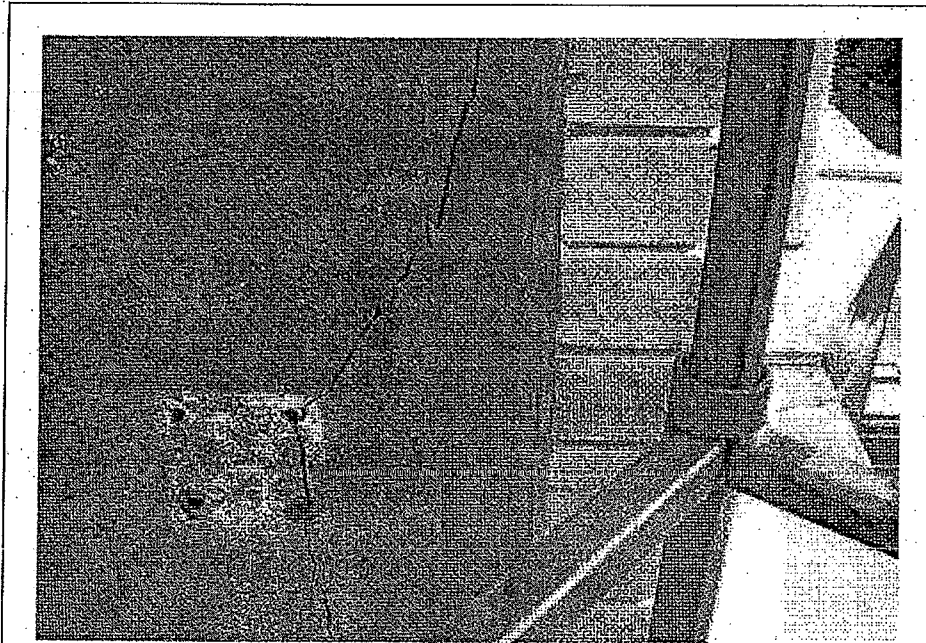
Figure B4-6: Rendered Beams & Columns – Damaged render columns on the northern wing.
