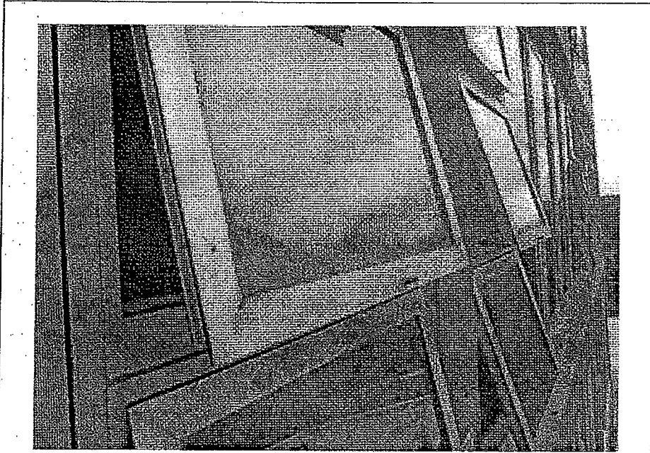
Figure B2-13: Windows and Louvres – Glazing film deterioration on new window panels on western wing.
