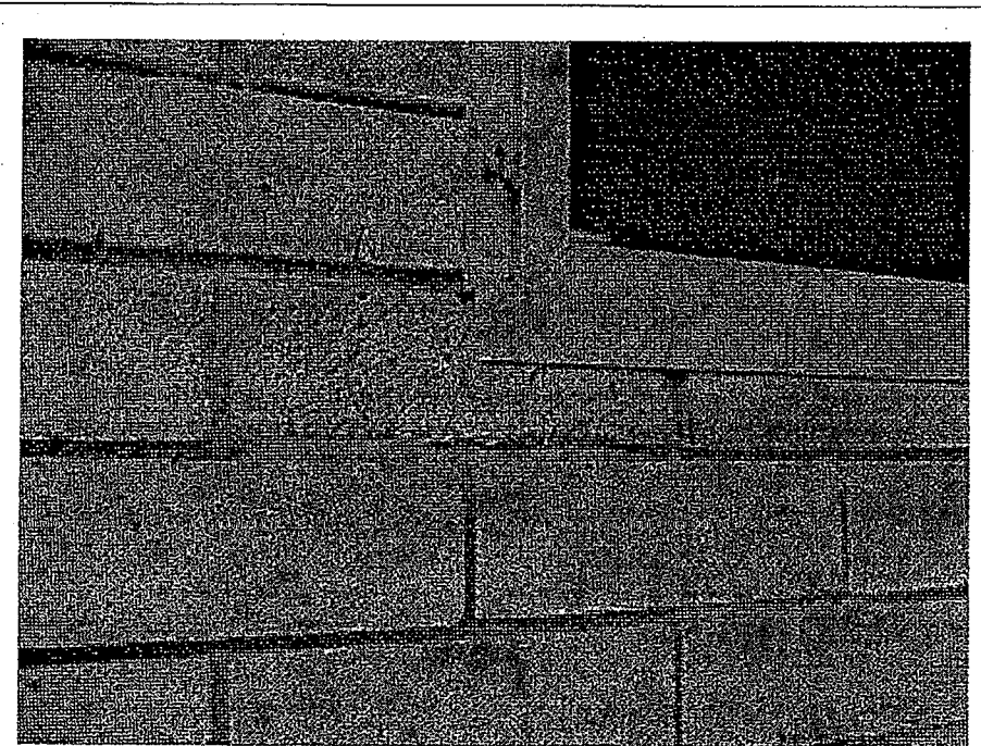
Figure B1-24: Brickworks – Surface erosion of brickwork (fretting).
