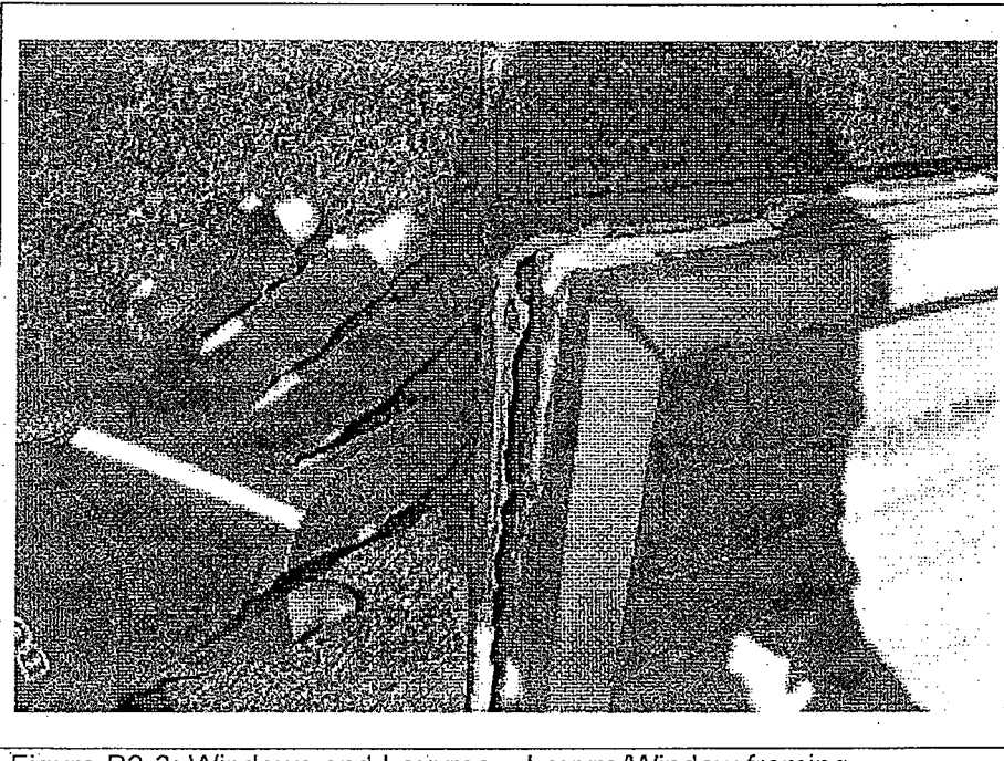
Figure B2-3: Windows and Louvres – Louvre/Window framing detachment from concrete structure and surface corrosion of louvres.
