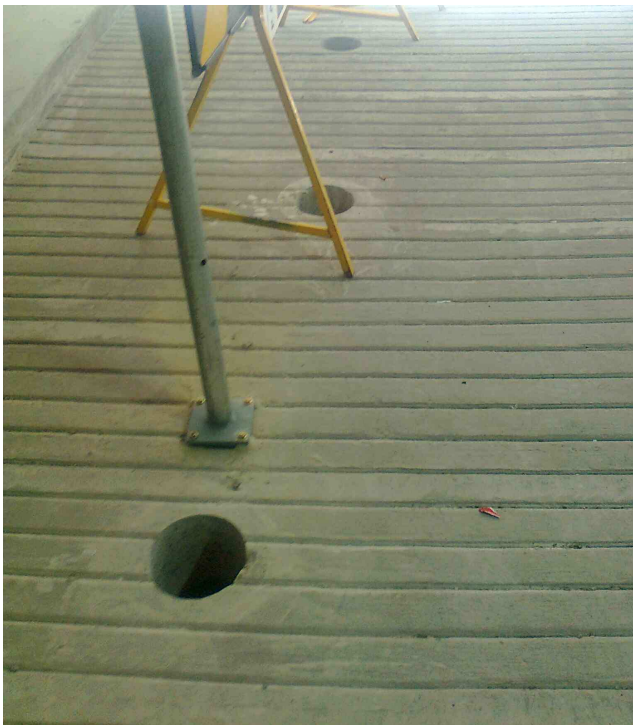
Bungan Lane Car Park – Photo shows the concrete slab entry / exit driveways was core drilled.
